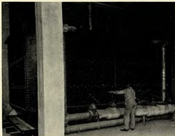
FIFTEEN THOUSAND GALLON HOUSE SUPPLY WATER TANK IN THE THIRTY-SECOND STORY
