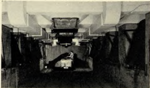
COAL CHUTES FROM OVERHEAD BUNKERS CONVEY COAL TO CARS ON INDUSTRIAL TRACK AND THENCE TO THE BOILERS
