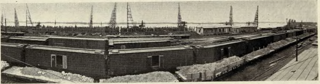
PANORAMIC VIEW LOOKING TOWARD SITE OF WHARFHOUSE, SHOWING CONDITION JANUARY 15, 1919. NOTE THE GREAT NUMBER OF PILES BEING DRIVEN TO SUPPORT THE WHARF AND WHARFHOUSE
