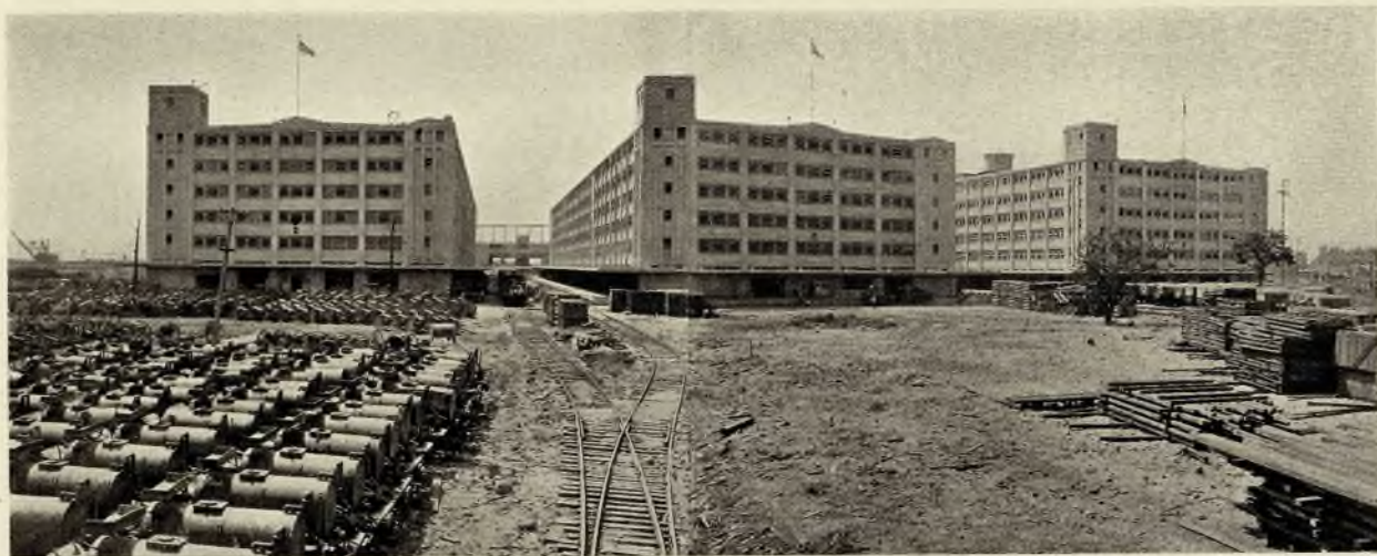
LANDSIDE VIEW OF COMPLETED WAREHOUSES. MATERIAL TO BE STORED SHOWN IN FOREGROUND. UNITED STATES ARMY SUPPLY BASE, NEW ORLEANS, LA. FORD, BACON AND DAVIS, SUPERVISING ENGINEERS. LIEUT.-COL. A. PEARSON HOOVER, Q. M. C., CONSTRUCTING QUARTERMASTER.
