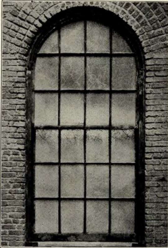
One of the round-headed windows which stood up excellently after a severe fire and high pressure water test.
