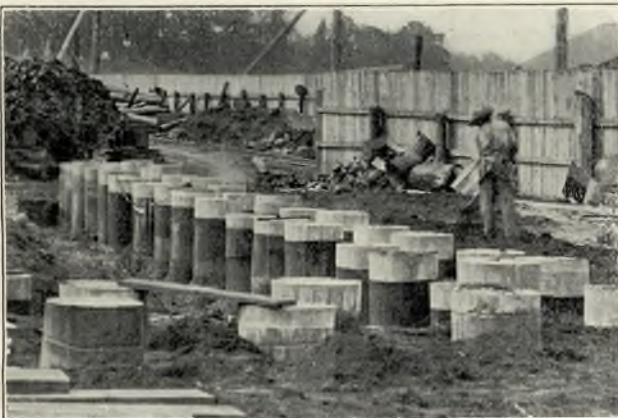
RAYMOND CONCRETE PILES IN FOUNDATION OF ACADEMIC BUILDING, UNITED STATES NAVAL ACADEMY, ANNAPOLIS, MD. ERNEST FLAGG, Architect
