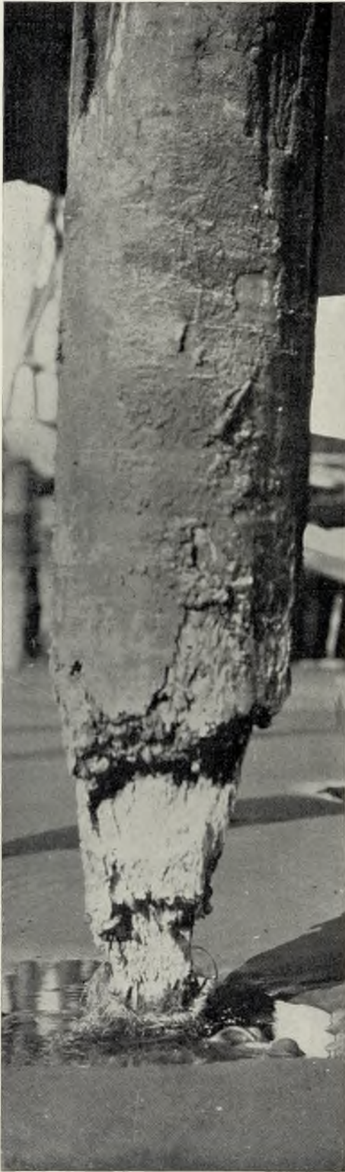
A Wood Pile on the Pacific Coast, showing the effects of teredos and limnoriae. Corrugated Concrete Piles are proof against such attacks.
